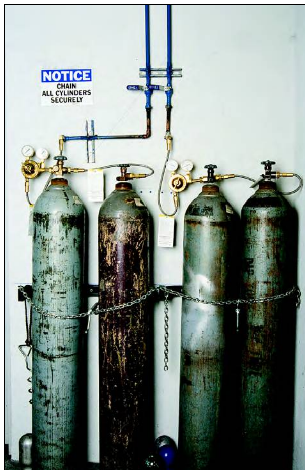
Figure 2.10—Inert Gas Cylinders Attached to Manifold System
