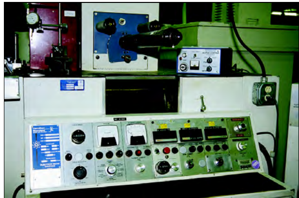
Figure 3.47—Electron Beam Welding Control Panel
