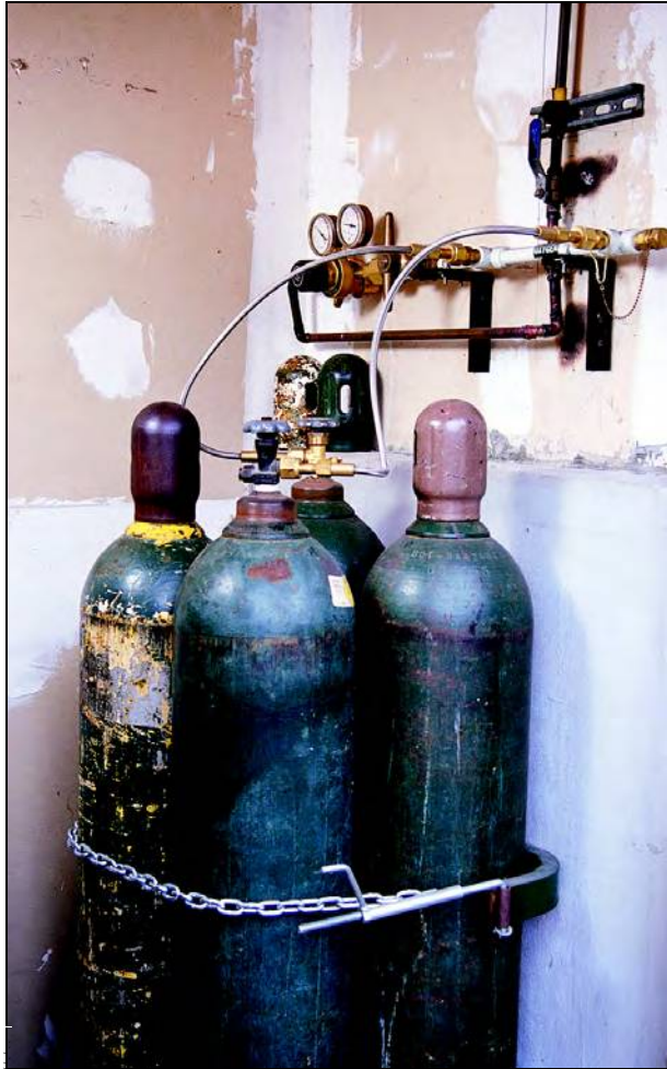
Figure 2.13—Oxygen Manifold System
